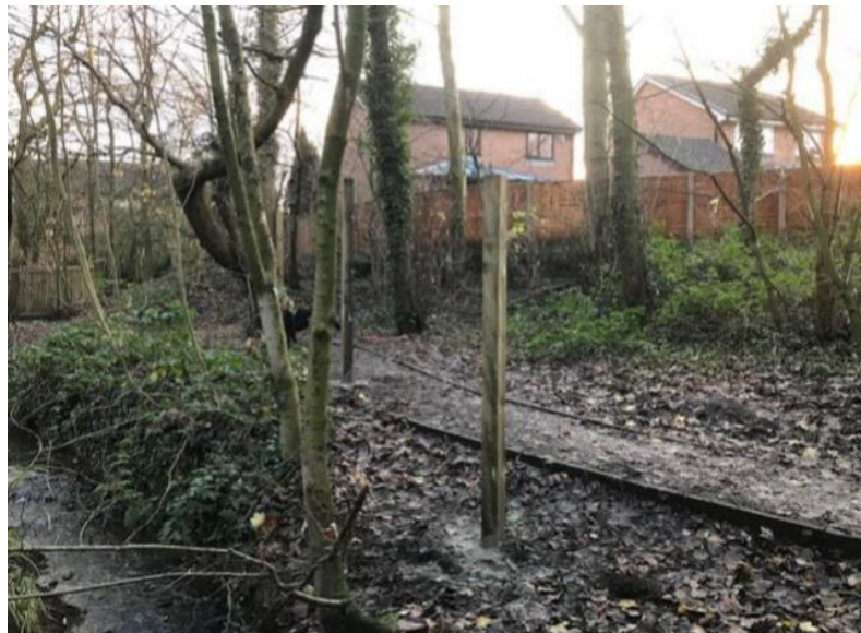
Further photograph showing the constructed path between point A and point B – November 2020
